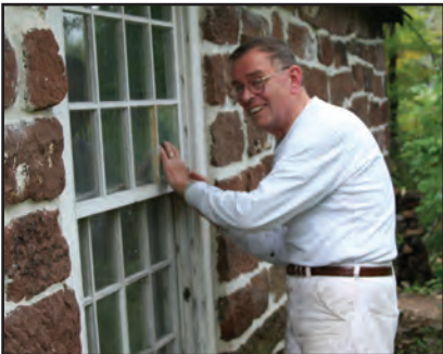
BCHS Member Manfred Wegner repairs broken window panes in the Out-kitchen and directed painting in the interior of the CC House.
